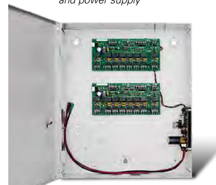
Two ELEV8 modules shown in enclosure with power supply
